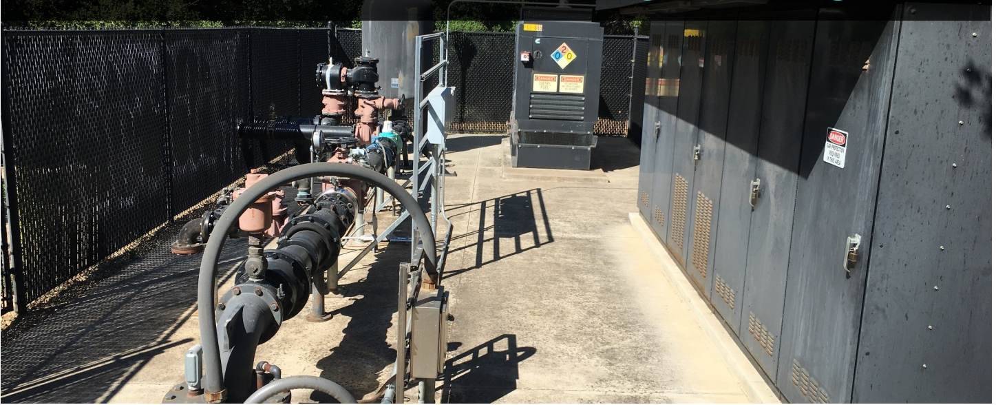
Pump station for stormwater capture at Stanford University
