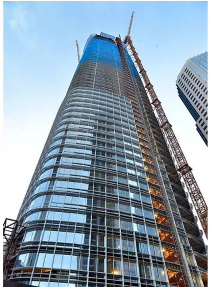
The Salesforce Tower in San Francisco has one of the largest onsite blackwater recycling systems in the world (Scott Hess)
