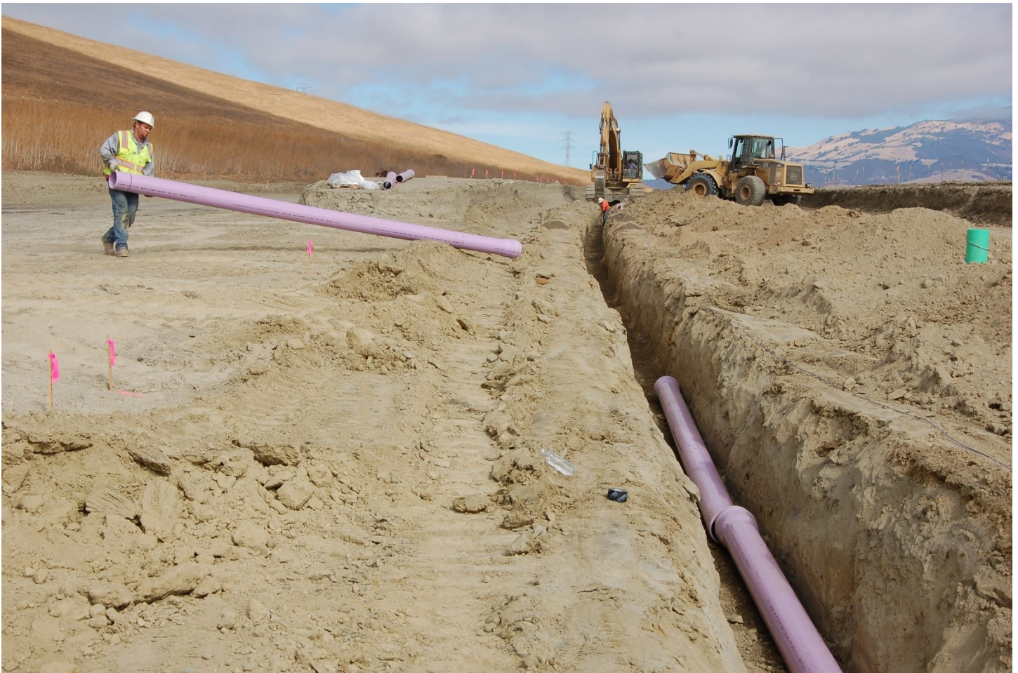
Purple pipes being installed to irrigate businesses and institutions in the San Ramon Valley Recycled Water program (Dublin, San Ramon and Pleasanton).
