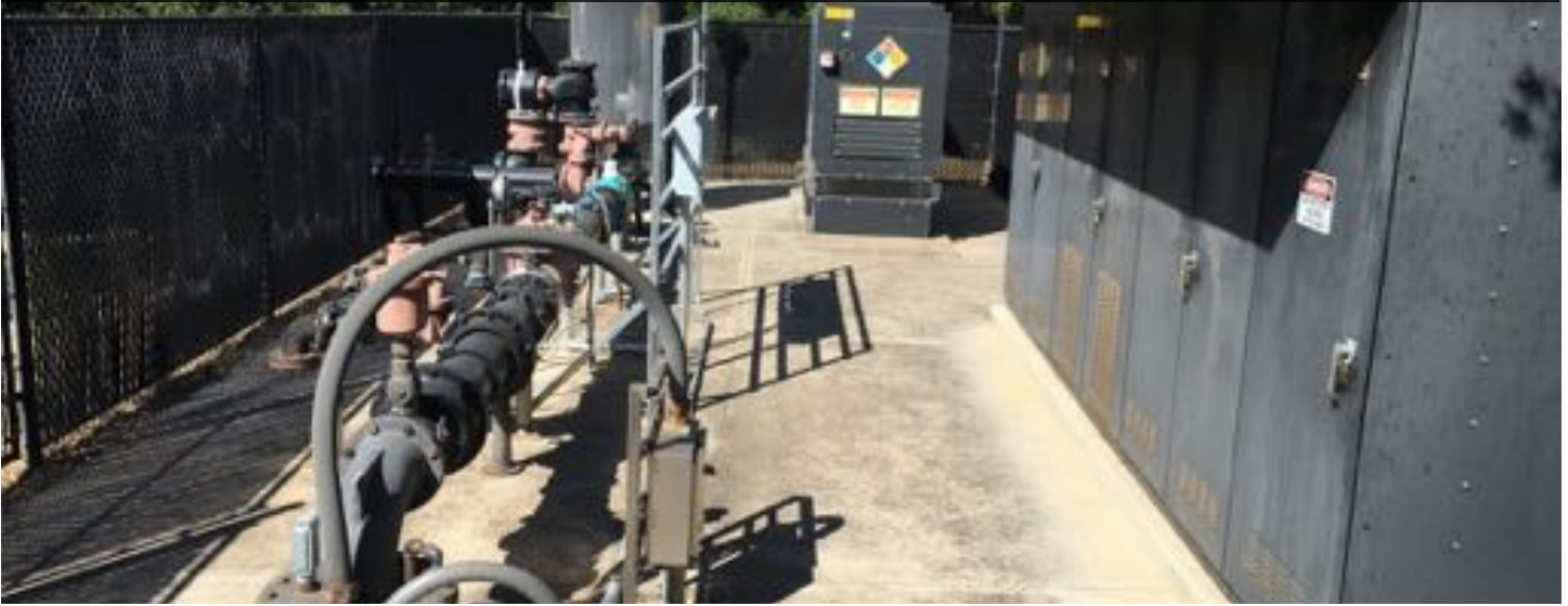
Pump station for stormwater capture at Stanford University
