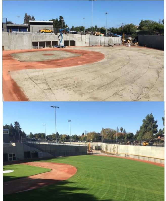
McKelvey Ball Park stormwater detention basin in Mountain View, during and after construction
