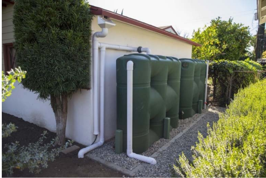
Figure 2-3. Roof runoff can be captured in rain barrels or cisterns to offset a small to moderate amount of potable water use.
