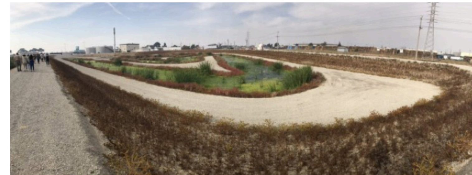
This so-called "horizontal levee" was built along the San Francisco Bay shoreline in a partnership with Oro Loma
